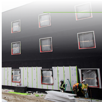
Indiana Law Enforcement Academy Plainfield, IN GreenGirt CMH XO System + SMARTci System
