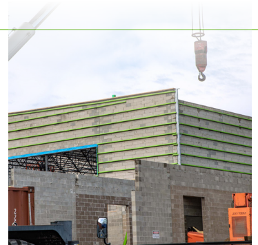
Mt. Hope Elementary School Lansing, MI GreenGirt CMH XO System + GreenGirt CMH System
